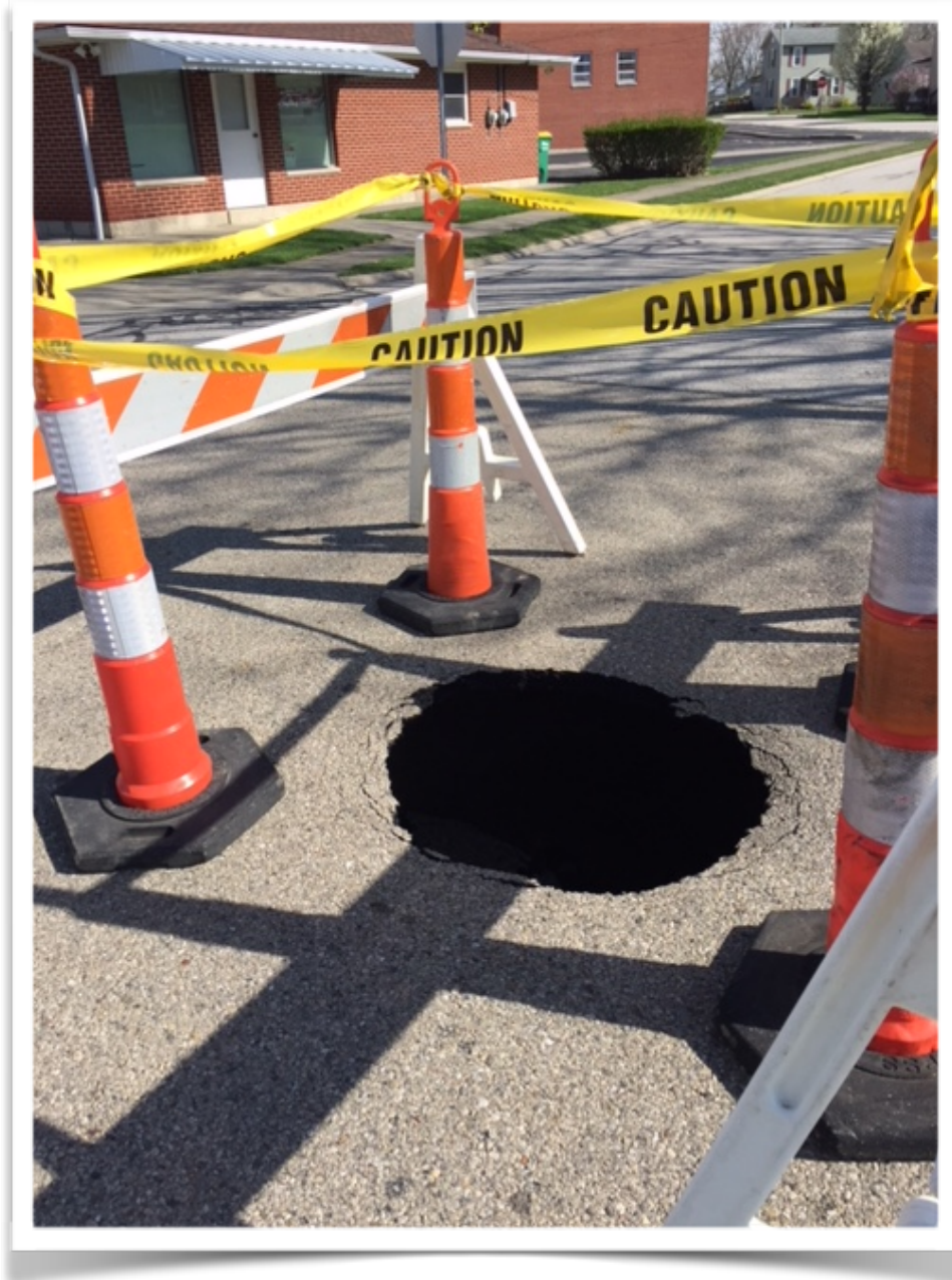
Sink hole at Clay and Church Streets.
