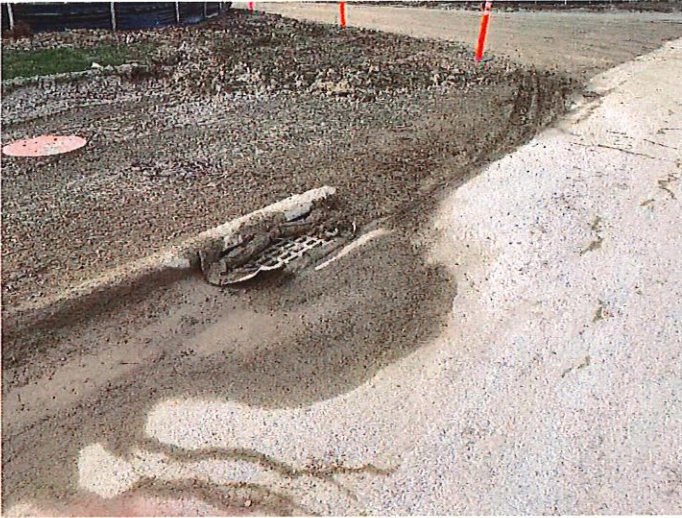
Eroded soil from rainwater drains down catch basin
